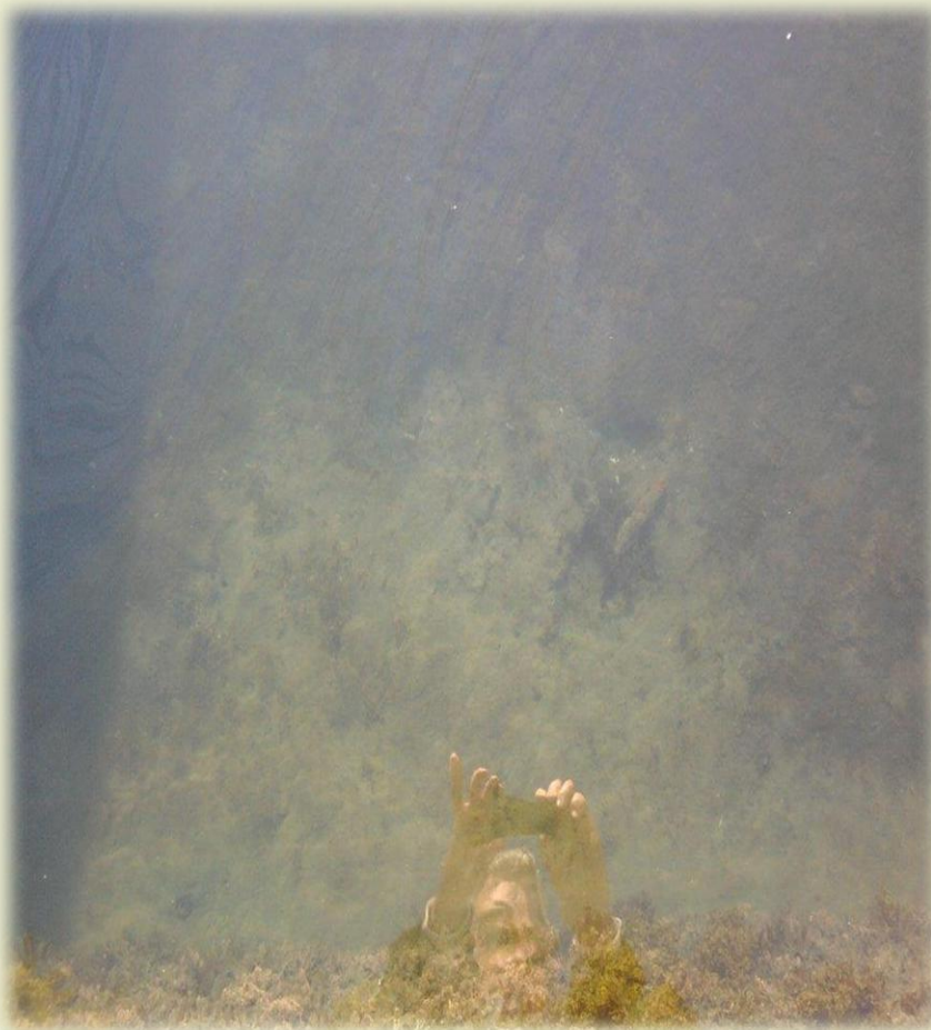
Bottom view through transparency - Before treatment concrete sill covered by sediments
